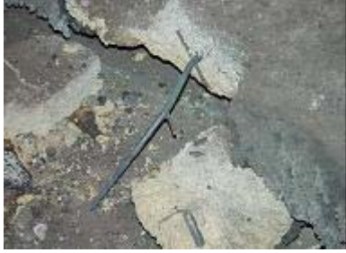
Fig. 1: Anchor attack and crack behaviour.
